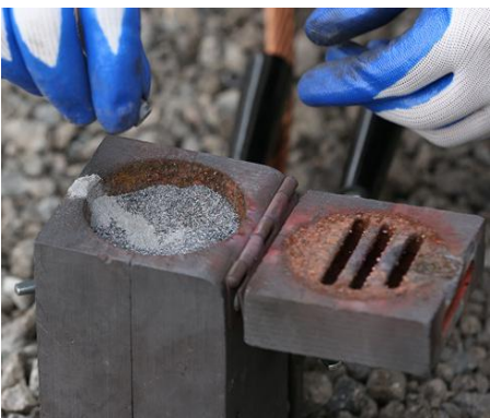
4. Sprinkle the starting powder over the weld powder and onto the lip of the mold. Close the cover.
