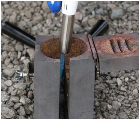
1. Position cleaned conductors in mold after making sure mold is dry, by pre-heating or making a test joint.
